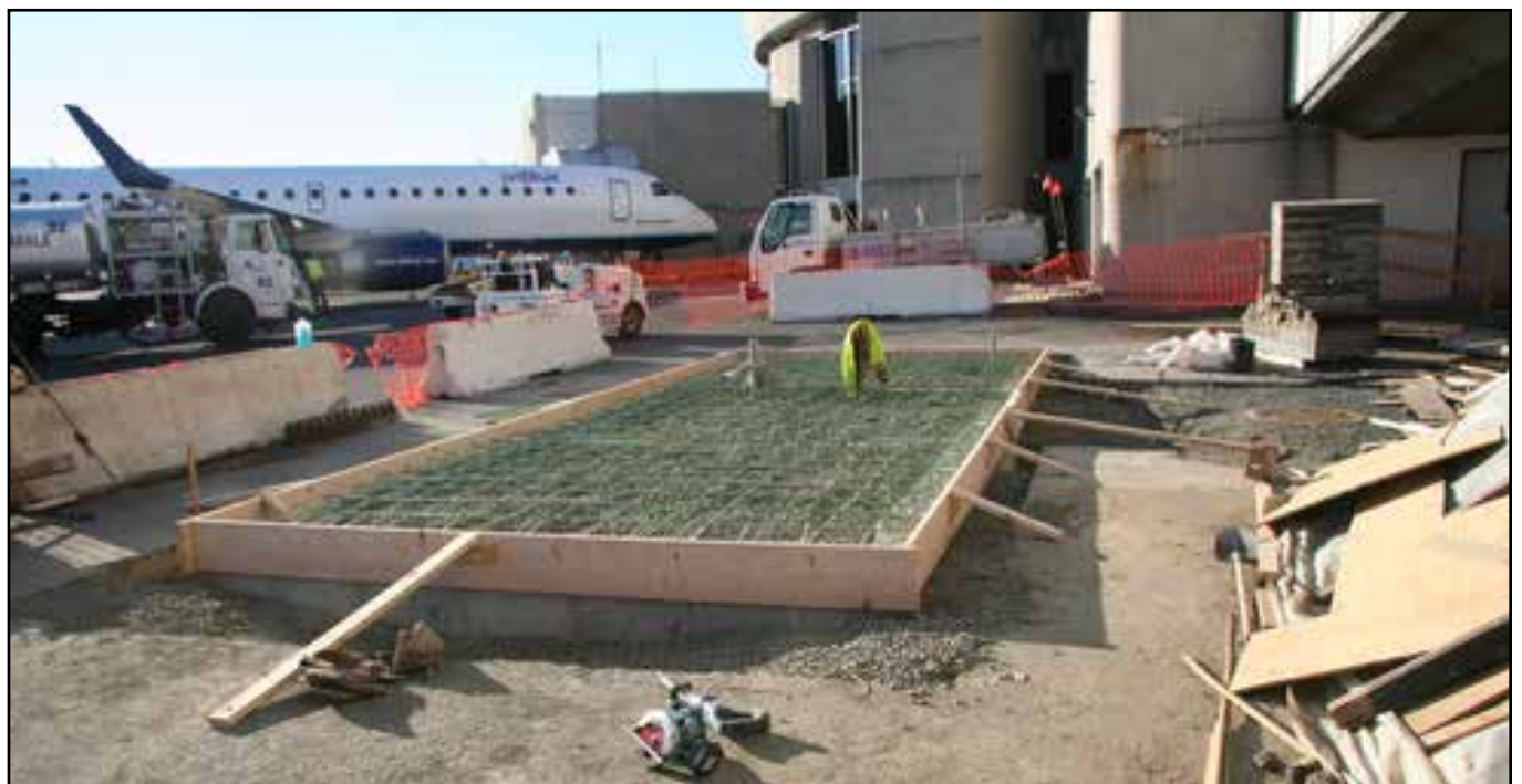
Reagan National Airport Combined Electrical System Upgrades
